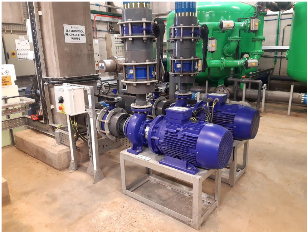
New Recirculating Pumps
