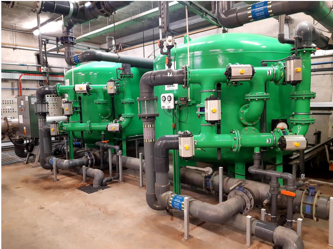
Refurbished Pressure Filters
