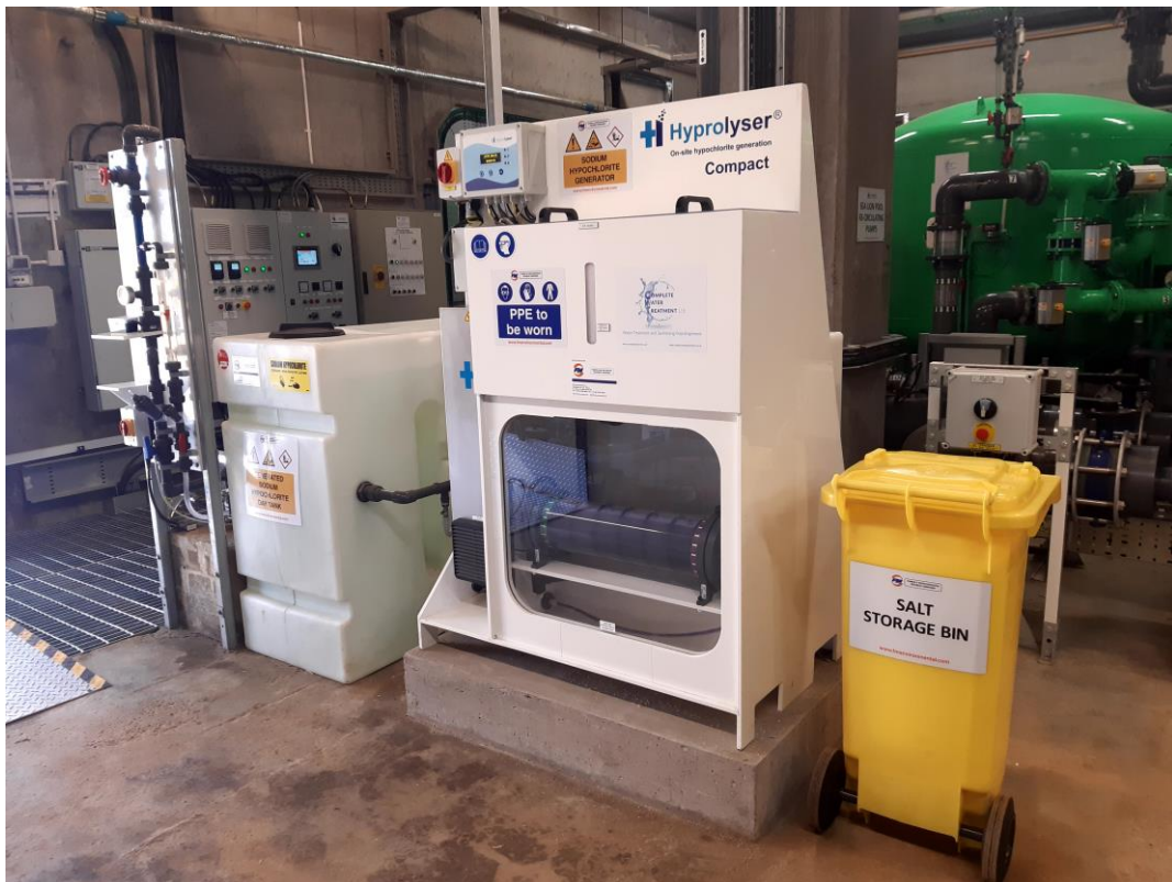
New Chlorine Generator, Day Tank and Dosing Unit
